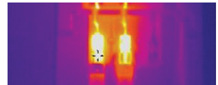
Electrical Predictive Maintenance Inspections & Troubleshooting
